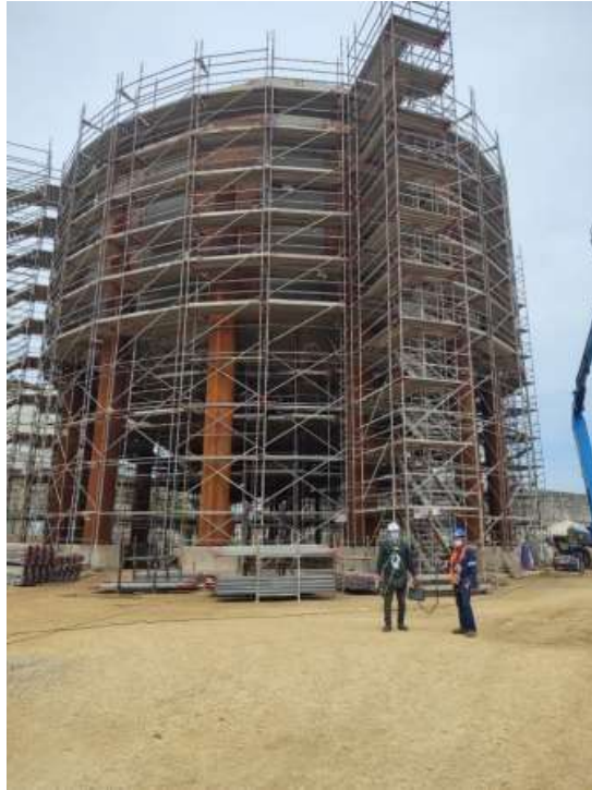
Figure 15 Spherical carbon steel tank located at the esenttia plant, Cartagena – Colombia
